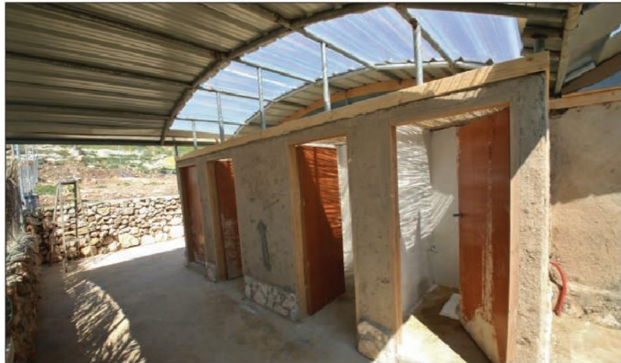
Public toilet have been improved. Shaded and with natural lighting and have been relocated closer to the main building.
