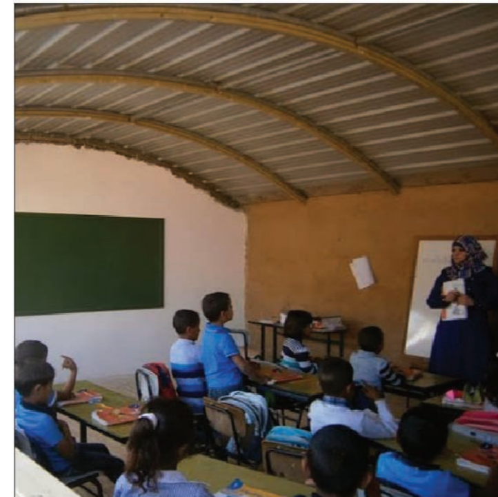
Al Ramadin new school under construction. The number of students has already increased. (6 classes, 6 teachers).
